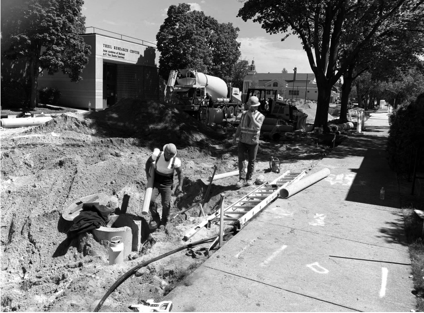
Part of our “unsettled” year involved the city’s reconstruction of Tenth Street, making the Theil Research Center almost inaccessible for several months. The road now features a north-side bike lane and south-side parking.
